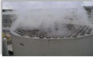
Boiler Blow off application
